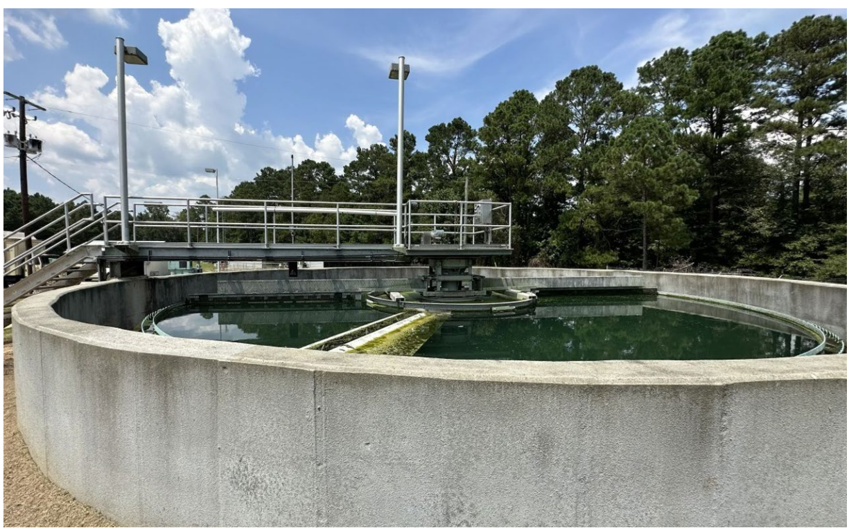
Eastover WWTP - Secondary Clarifier
