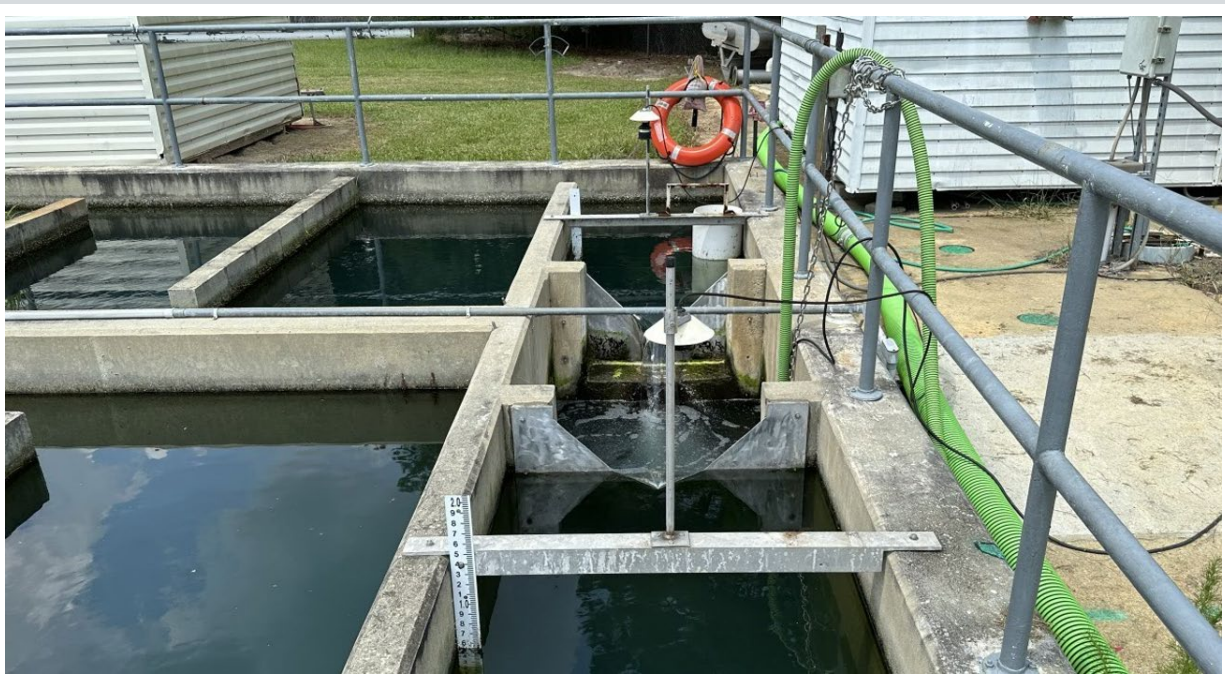
Eastover WWTP - Chlorine Contact Chamber and Flow Measurement
