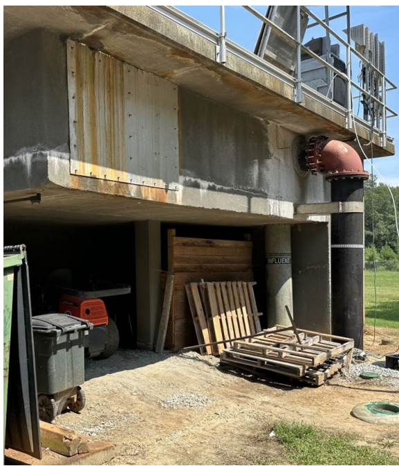
Eastover WWTP - Influent Piping at Headworks
