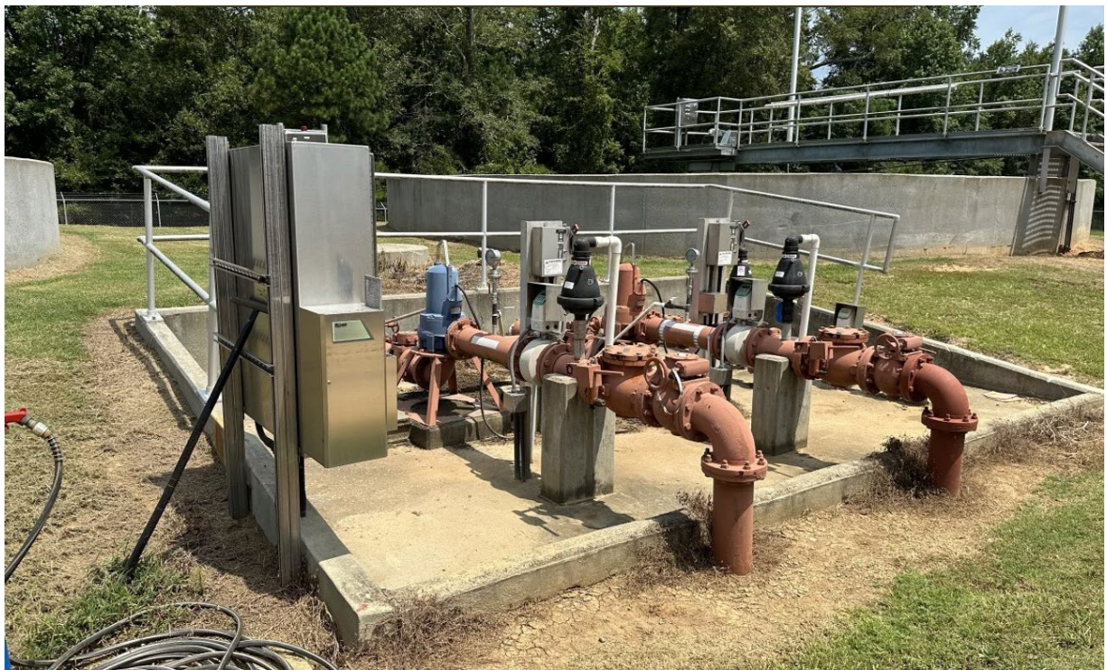
Eastover WWTP - RAS/WAS Pump Station
