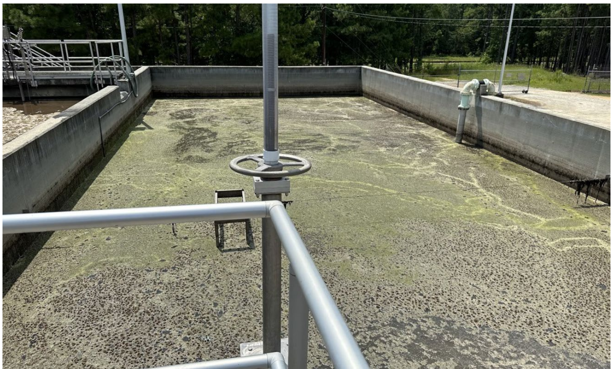
Eastover WWTP - Aerobic Digester
