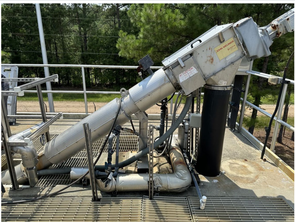
Eastover WWTP - Headworks Screening
