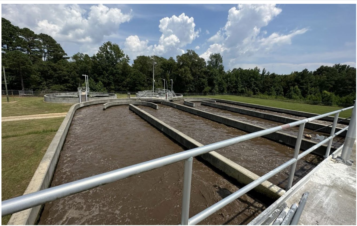
Eastover WWTP - Aeration Basins
